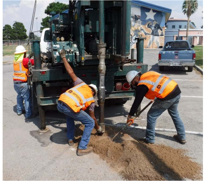
PHOTO NO. 22: General view of drilling activities at exploration soil boring 2B-29 location.
