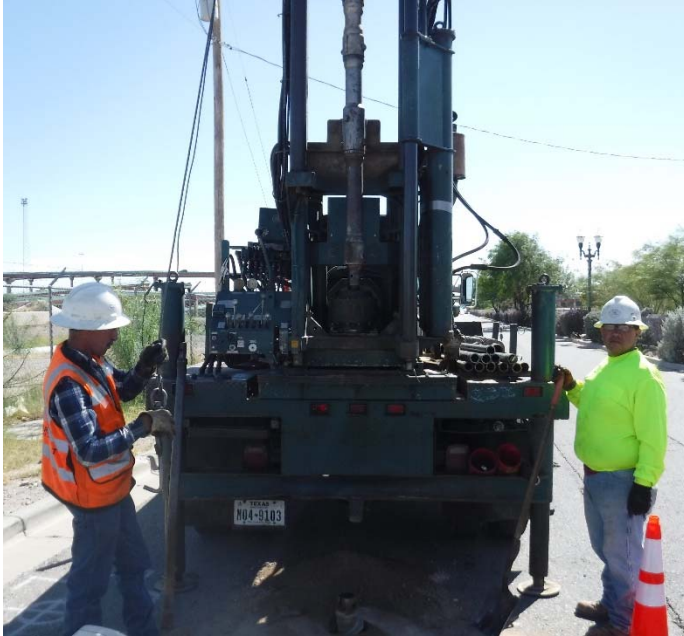
PHOTO NO. 9: General view of drilling activities at exploration soil boring 2B-1 location.
