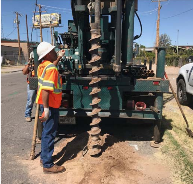
PHOTO NO. 17: General view of drilling activities at exploration soil boring 2B-13 location.
