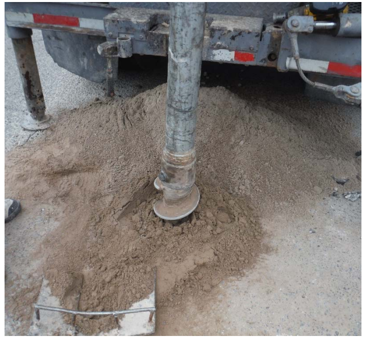
PHOTO NO. 8: General view of drilling activities at exploration soil boring B-7 location.
