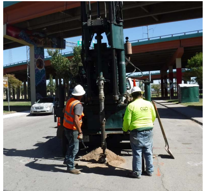
PHOTO NO. 12: General view of drilling activities at exploration soil boring 2B-5 location.
