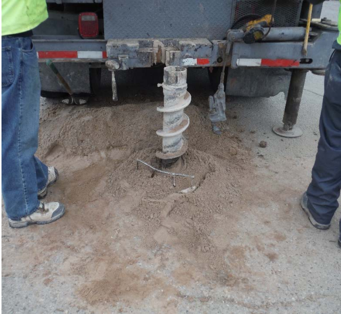
PHOTO NO. 5: General view of drilling activities at exploration soil boring B-4 location.
