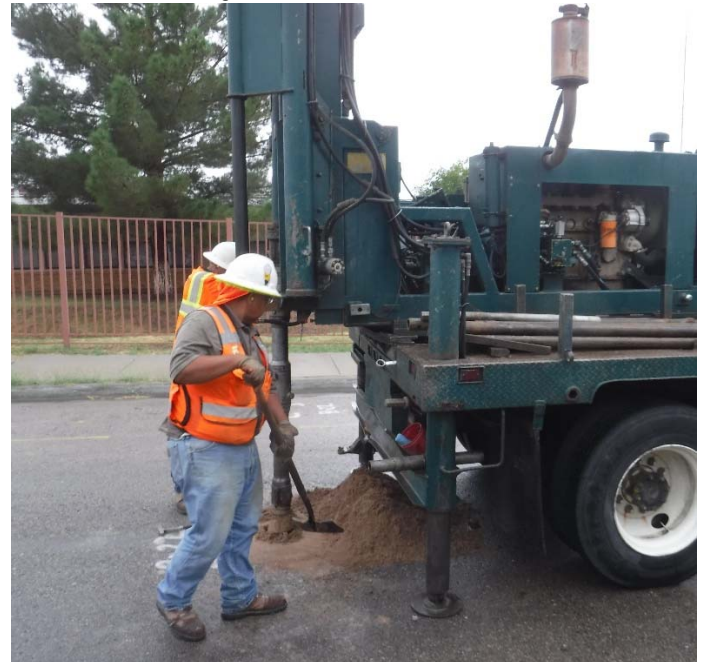
PHOTO NO. 20: General view of drilling activities at exploration soil boring 2B-22 location.
