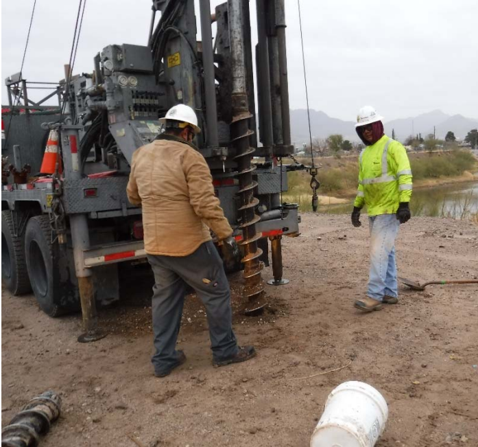
PHOTO NO. 1: General view of drilling activities at exploration soil boring B-1 location.
