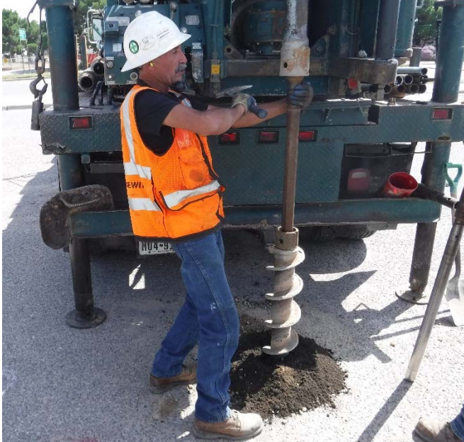
PHOTO NO. 21: General view of drilling activities at exploration soil boring 2B-28 location.
