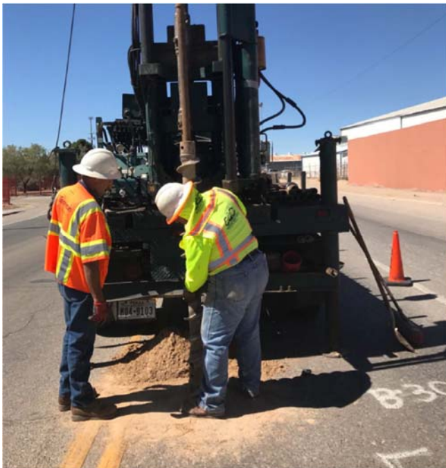
PHOTO NO. 23: General view of drilling activities at exploration soil boring 2B-30 location.
