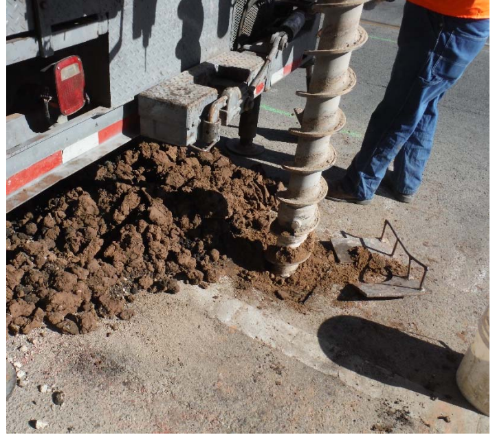
PHOTO NO. 6: General view of drilling activities at exploration soil boring B-5 location.
