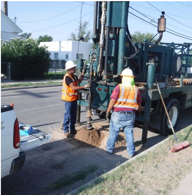
PHOTO NO. 19: General view of drilling activities at exploration soil boring 2B-20 location.
