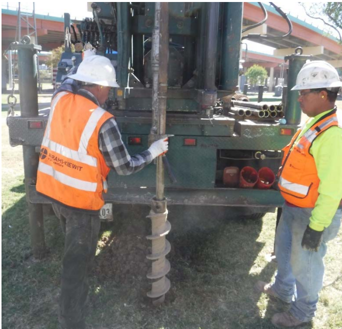
PHOTO NO. 11: General view of drilling activities at exploration soil boring 2B-4 location.
