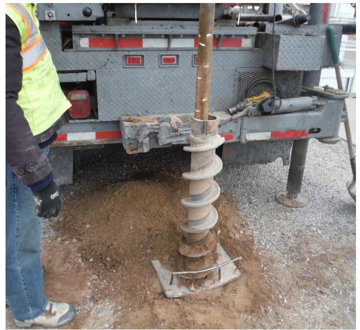
PHOTO NO. 4: General view of drilling activities at exploration soil boring B-3 location.
