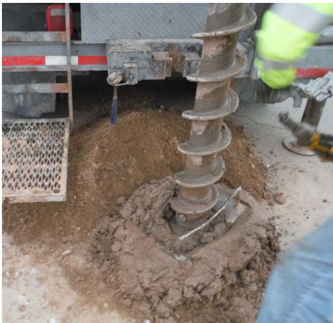
PHOTO NO. 7: General view of drilling activities at exploration soil boring B-6 location.
