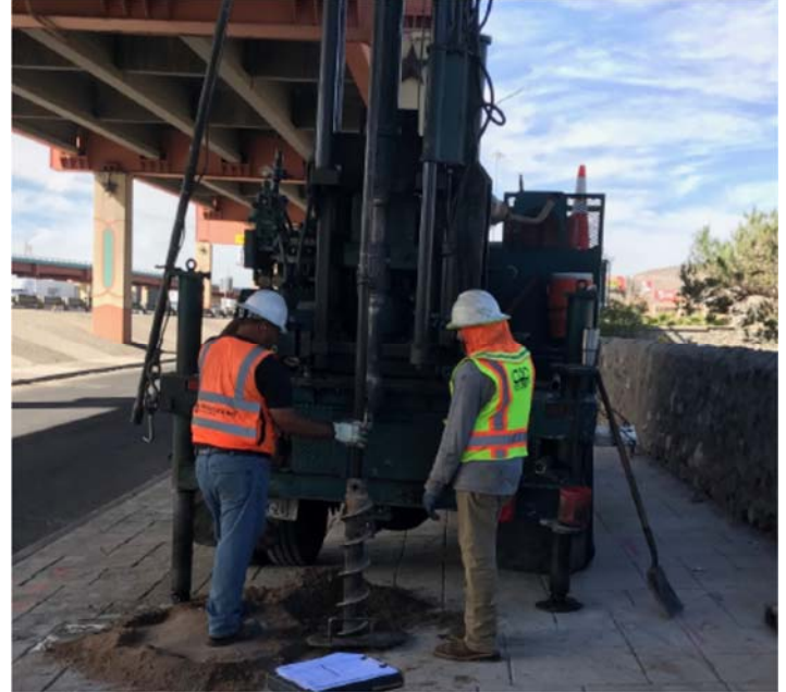
PHOTO NO. 10: General view of drilling activities at exploration soil boring 2B-3 location.
