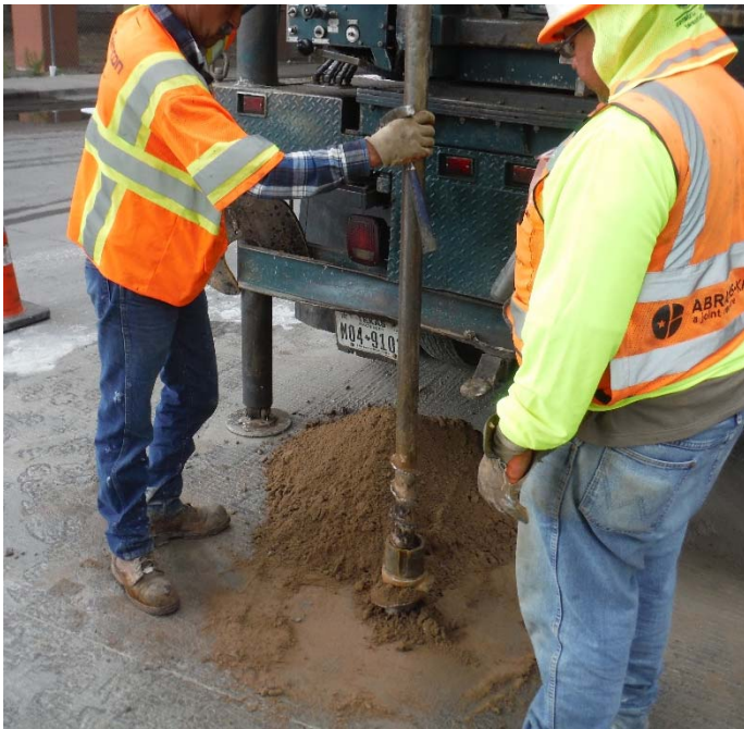
PHOTO NO. 15: General view of drilling activities at exploration soil boring 2B-10 location.
