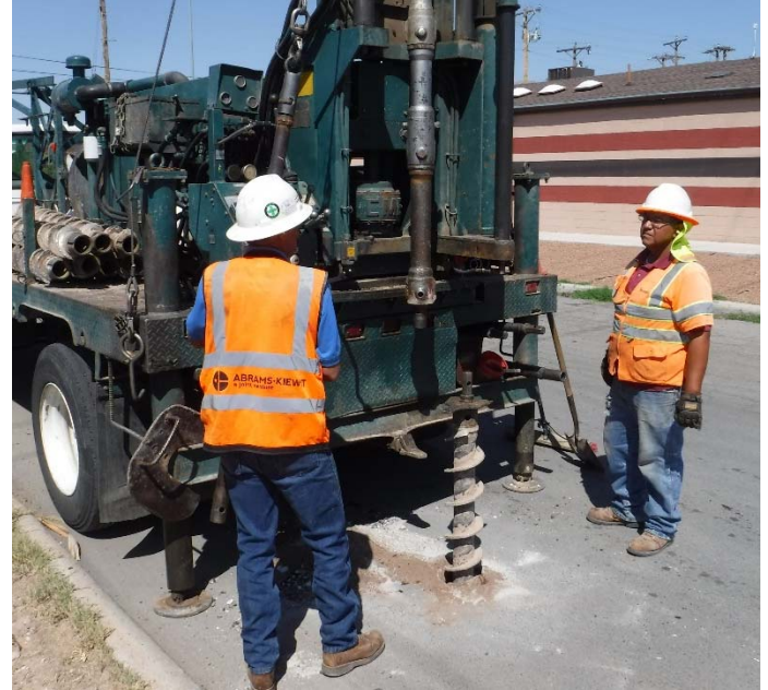
PHOTO NO. 18: General view of drilling activities at exploration soil boring 2B-16 location.
