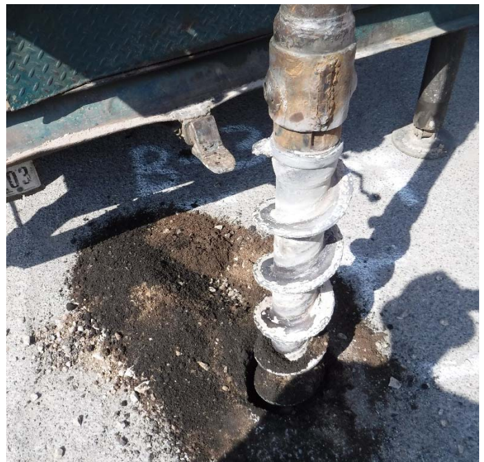
PHOTO NO. 24: General view of drilling activities at exploration soil boring 2B-34 location.
